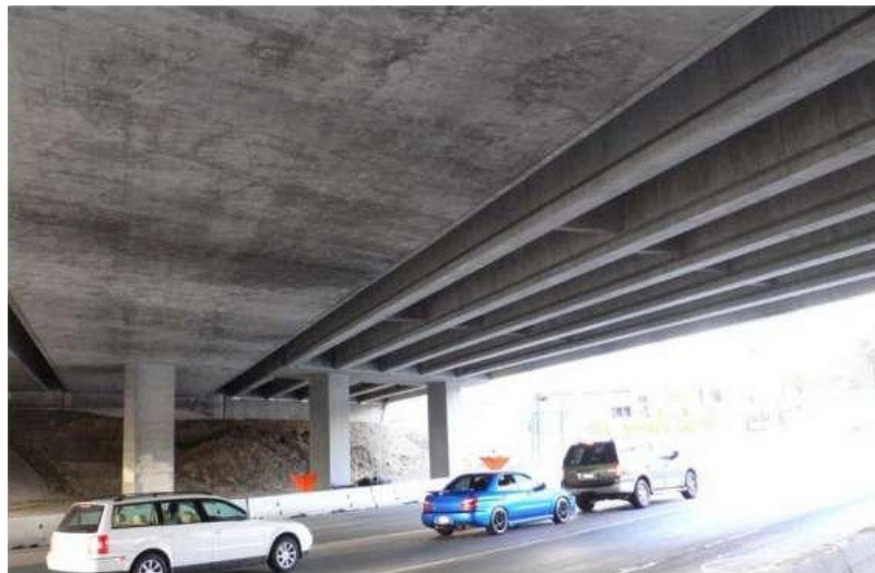
Figure 1.2. Example of the use of precast I-girders on a highway bridge widening project in California. (International Federation of Structural Concrete, 2007)
